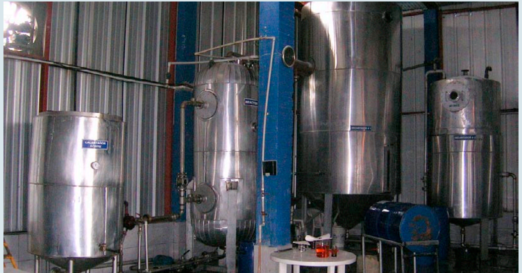
A plant for the conversion of fish waste into biodiesel.
